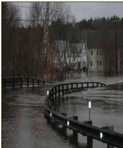
Main Street bridge near downtown Raymond during the April 2007 flood event.
